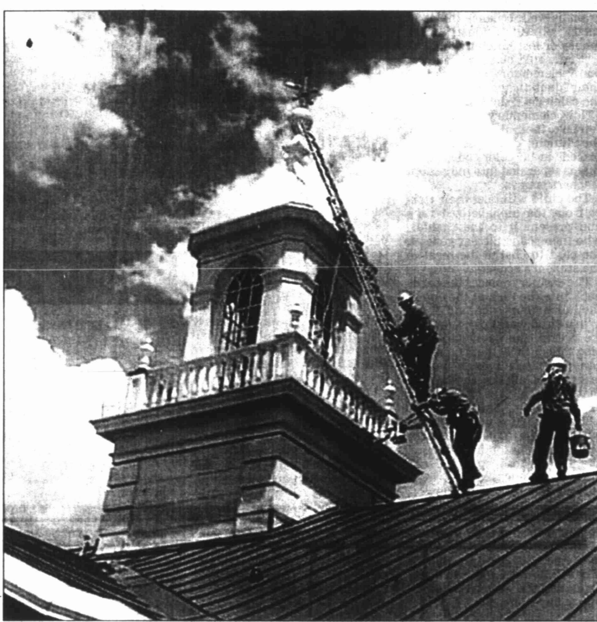
Workmen with the Seyforth Co. of El Paso scale the steeple of the administration building of Big Spring State Hospital to paint the picturesque landmark. The steeple work is just a part of a major construction project putting new metal roofs on eight of the hospital's buildings. The project began in December and is expected to be completed in September.
