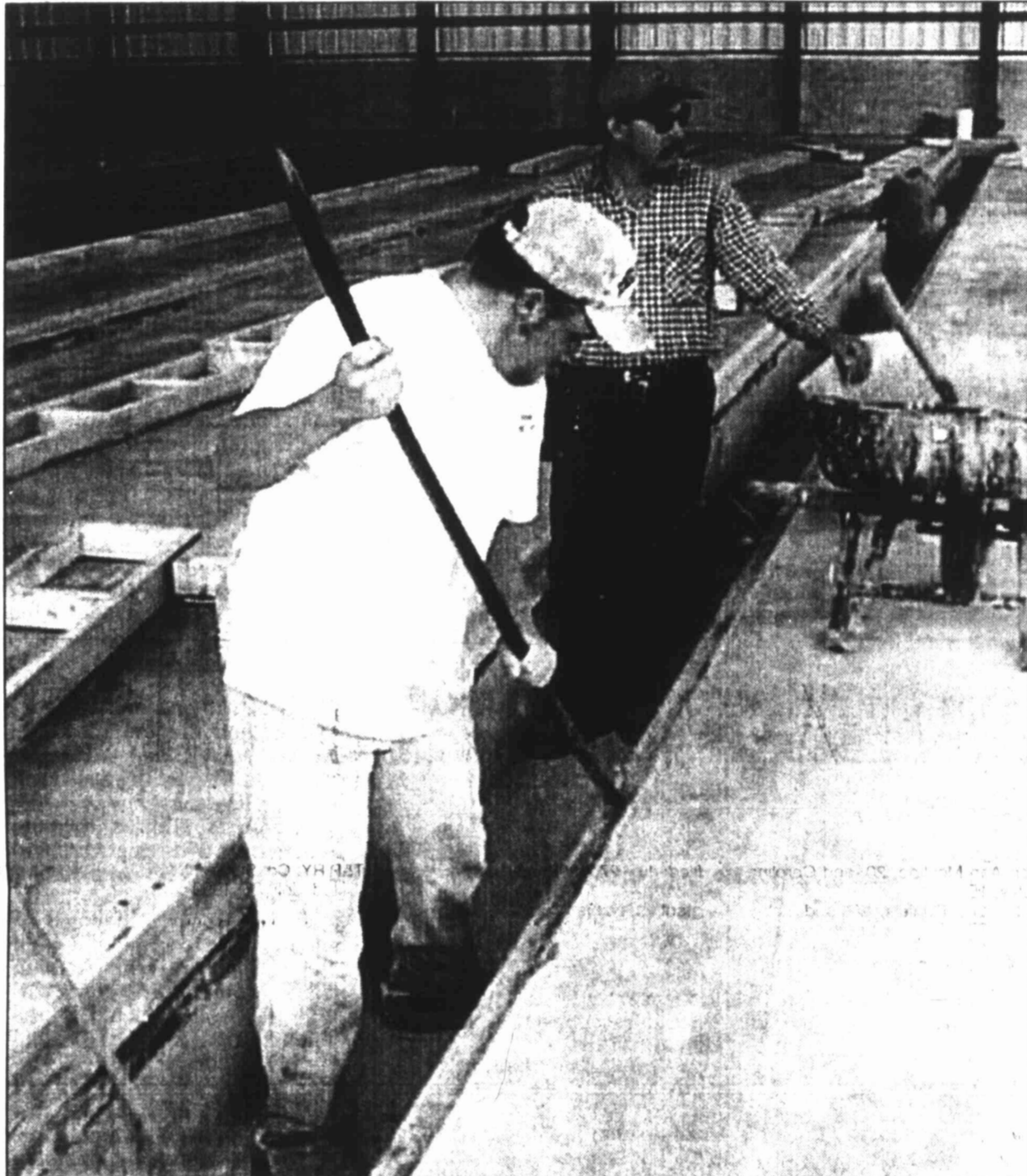
Ben Chester and Juan Garcia of Abco Builders, Midland, finish the aeration tunnels of the new 32,000 square foot seed storage warehouse at Stoneville, Texas.
