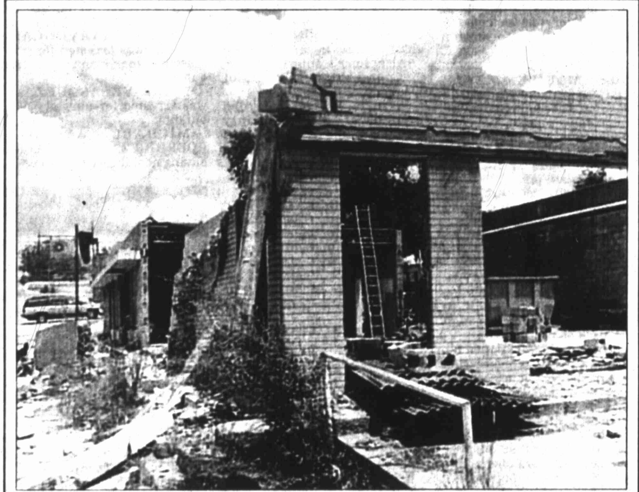
A building on Ninth Street near downtown Big Spring is in the process of being demolished. The city has an on-going program for tearing down dilapidated and abandoned buildings.
