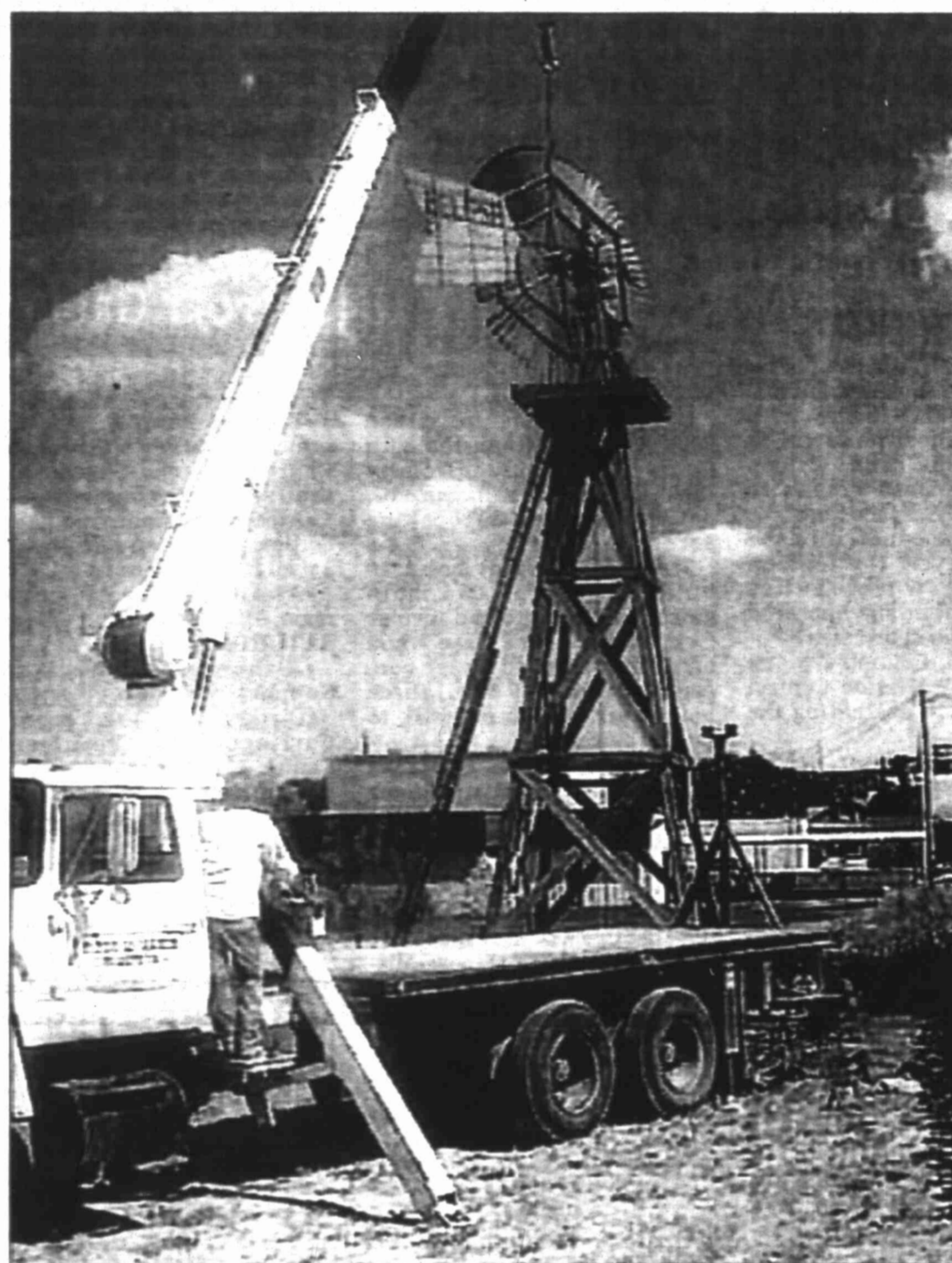
The turn-of-the-century Eclipse windmill at The Heritage Museum of Big Spring was reassembled Thursday with the help of a mobile crane following painting and maintenance for the windmill's turbine. Doing the tower work was Ron Hale. Boosie Weaver was in charge of the historic windmill restoration project. Clyde McMahon Concrete donated the time for the crane truck and operator Leland Gullatt. The Eclipse windmills made it possible to ranch in arid climates more efficiently. The wooden windmills were replaced by metal windmills about 1920.
