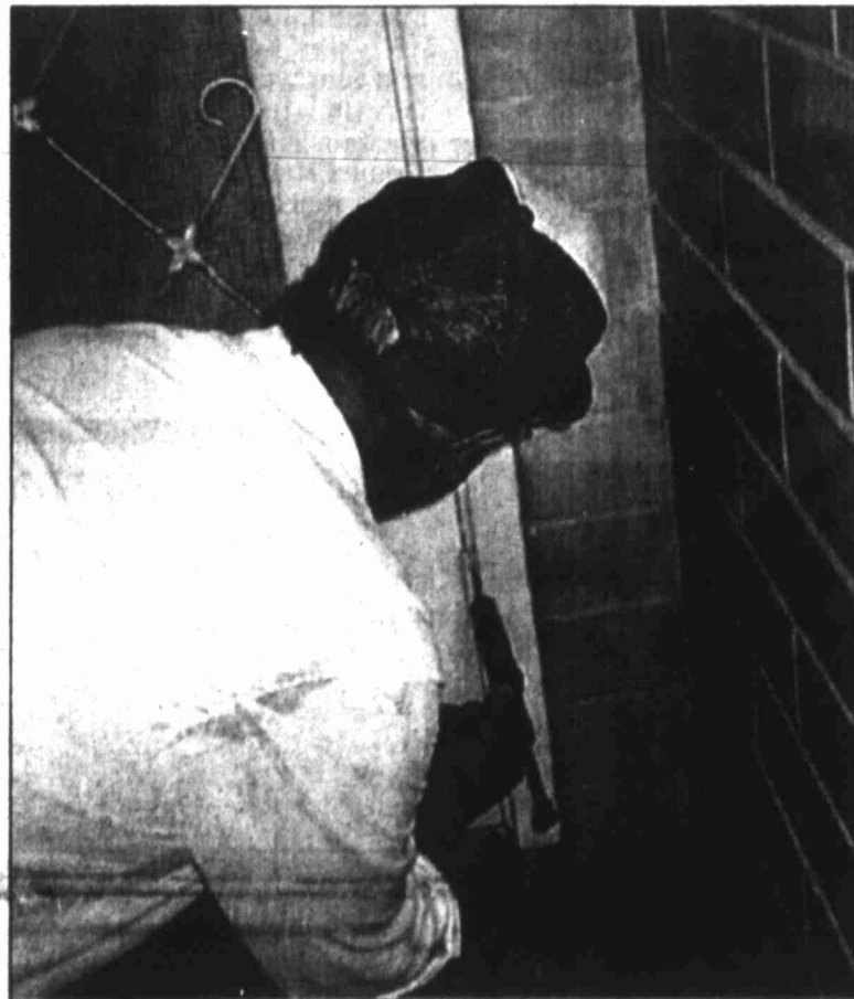
Far left, Jerry Dean, who has 18 years in the pest control business with Southwestern A-1 Pest Control, sprays corners and other favorite areas of bugs at St. Mary's Episcopal School. Left, Dean applies a chemical bait to cracks behind a door. Dean was doing the school's routine pest control treatment last week. Below, left, Dean mixes chemicals into a sprayer before going to work inside the school. Below, Dean uses "glue boards" to attract and trap insects in areas where spraying insecticide is not safe, such as kitchens.
