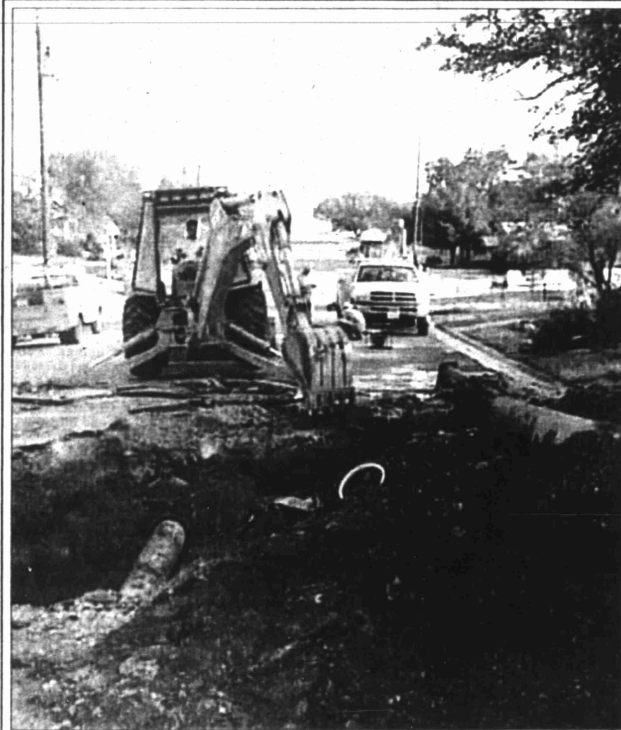
City repairmen were busy repairing another transmission line break this morning, this one on Lancaster between 10th and 11th. John Martinez is operating the heavy equipment. The city started experiencing breaks Friday afternoon, said Todd Darden, director of community development. Primary breaks were at 16th and Virginia and 12th and Lancaster.
