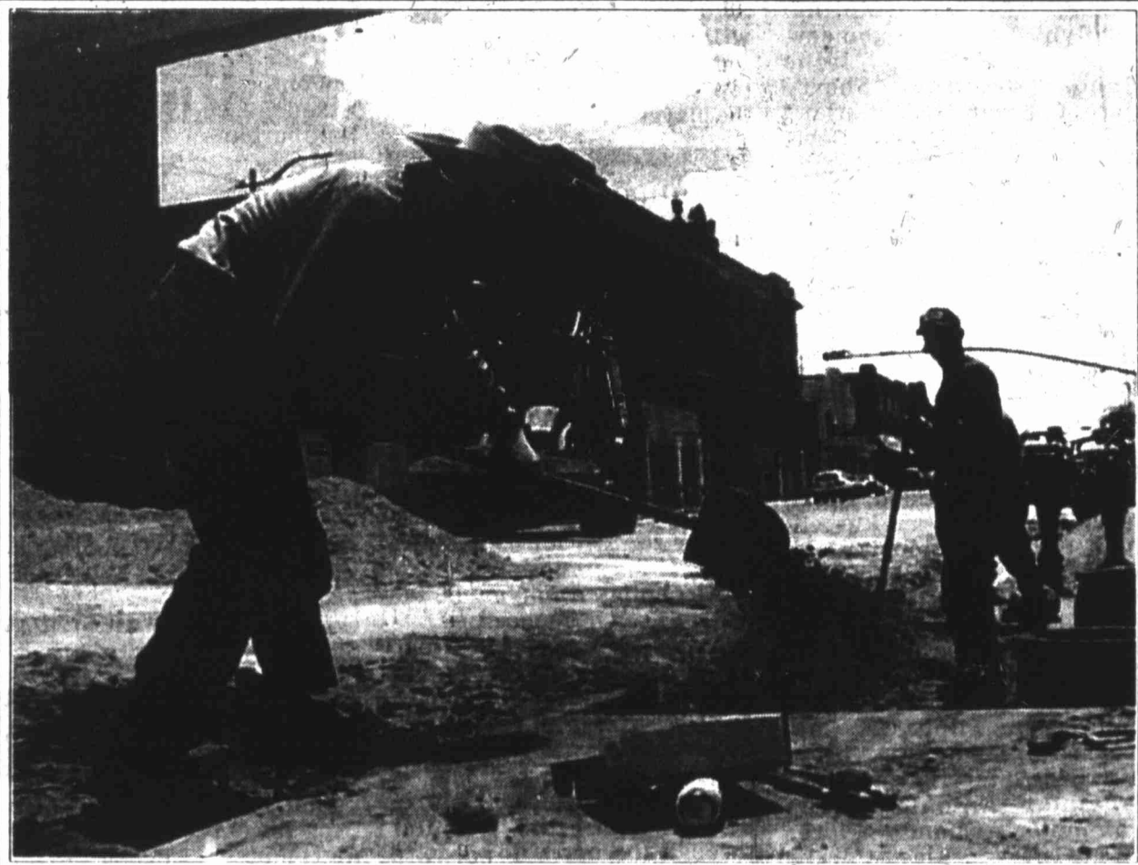
City water department employees Michael Sizenback (left) and James Dalley fill in the hole after city employees replace an 8-inch water line on Third Street, directly across from the Settles Building. Seventy-two feet of water line was replaced on the project last Thursday and Friday.
