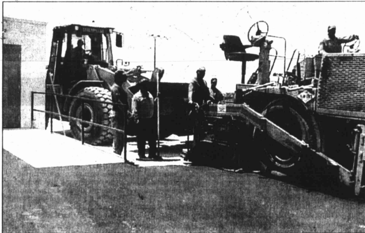
Price Construction crews worked all last week to grade and pave the area east of the new restroom facility at the Big Spring Rodeo Bowl. As many as 45 men worked to have their project completed before the rodeo begins Wednesday. Pictured are Junior Herrera, left, Randy Price, Joey Loper, Jesse Ferrel in the loader, Catriño Guerrero, Cynthia Galley, lab, and Tim Atkins, mechanic.
