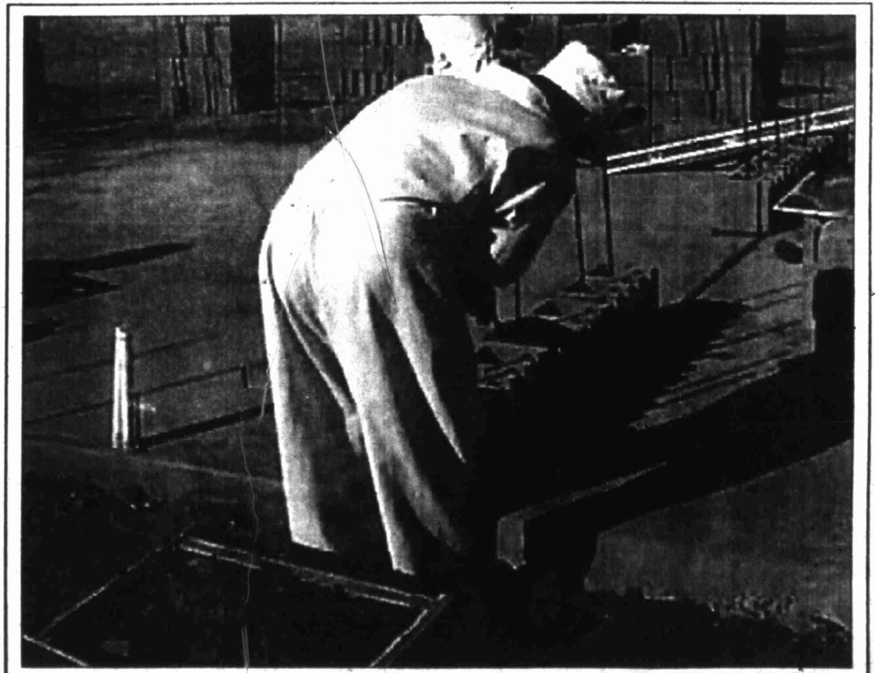
Inmates from the Big Spring Wilderness Camp began construction on the chapel at the Big Spring Vietnam Memorial this morning. Work is expected to take three days.
