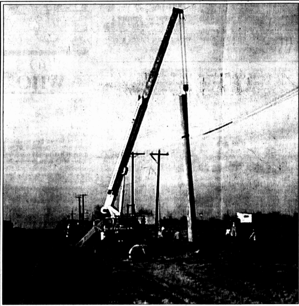
Hotline Utility Construction of Stanton, erects poles near the intersection of FM 700 and U.S. Highway 87.
