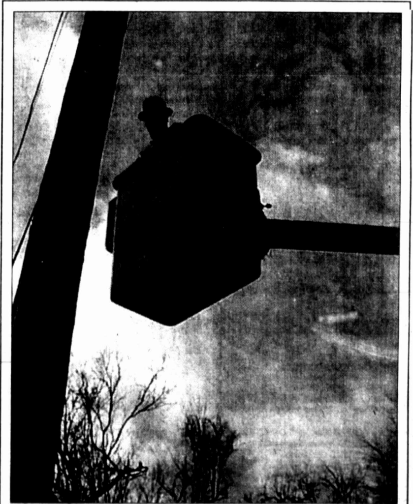
Bobby Joe Tucker with Cline Construction rips out old telephone wires along 8th Street
