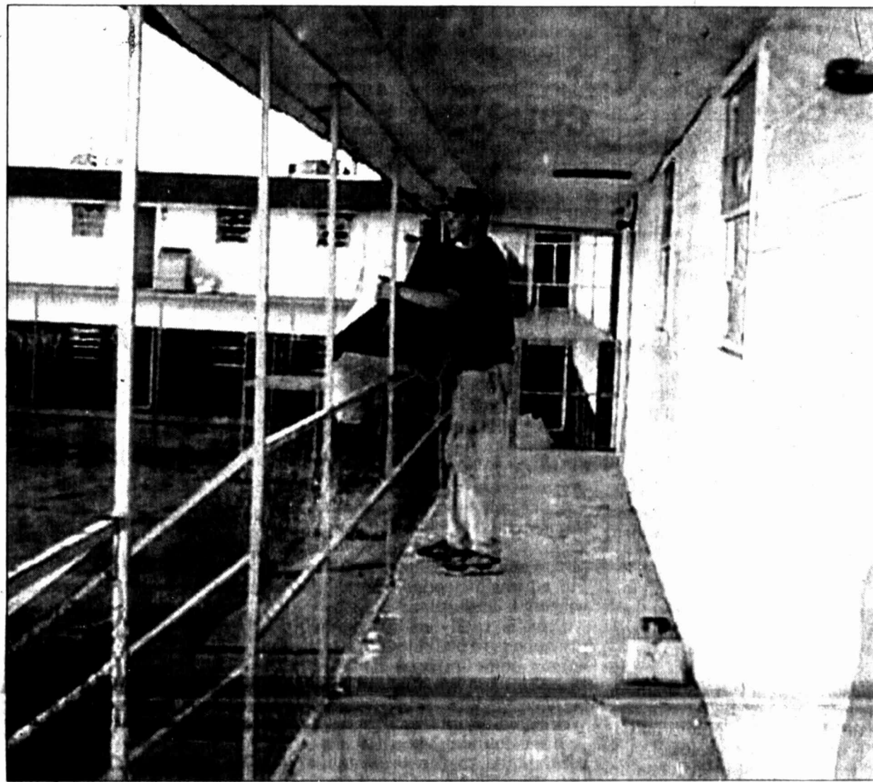
Brad Gibbs, working with Gibbs Remodeling, works to remove old carpet from the Western Hills Apartment complex, which is being refurbished and will provide additional housing in Big Spring.
