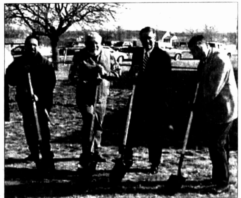
Arthur Palomino, Johnny Cappadonna, Jack Swallow and Max Webb break ground for the basketball court lighting project at the Northside Community Center. Palomino is vice-president of the center's advisory board, while Webb is the executive director. Cappadonna's Capp Electric will do the work and Swallow is executive director of the Permian Basin Foundation, which helped fund the project.
