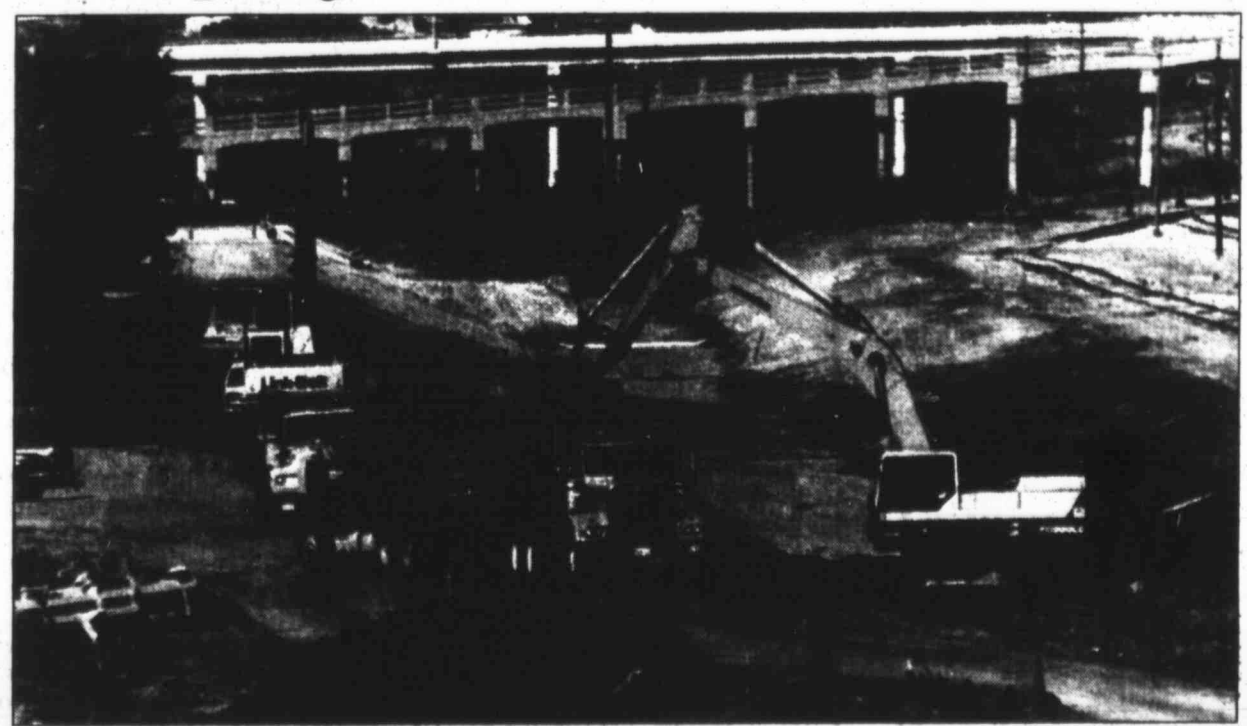
HERALD photo Decades in the planning and construction, the Beals Creek Flood Control Project was completed earlier this month.
