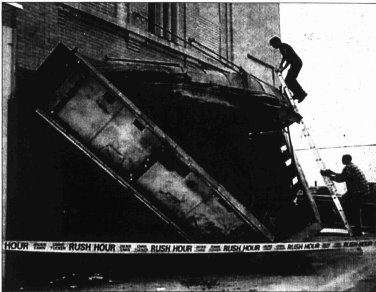
HERALD photo/Linda Choate Rocky Salzar and Aaron Bristow prepare the marquee of the Ritz Theater for removal. It is part of an extensive renovation project planned by the owner.
