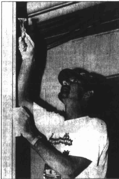
Keith Burrows of Big Spring completes finish work on the new dorms at the SouthWest Collegiate Institute for the Deaf.
