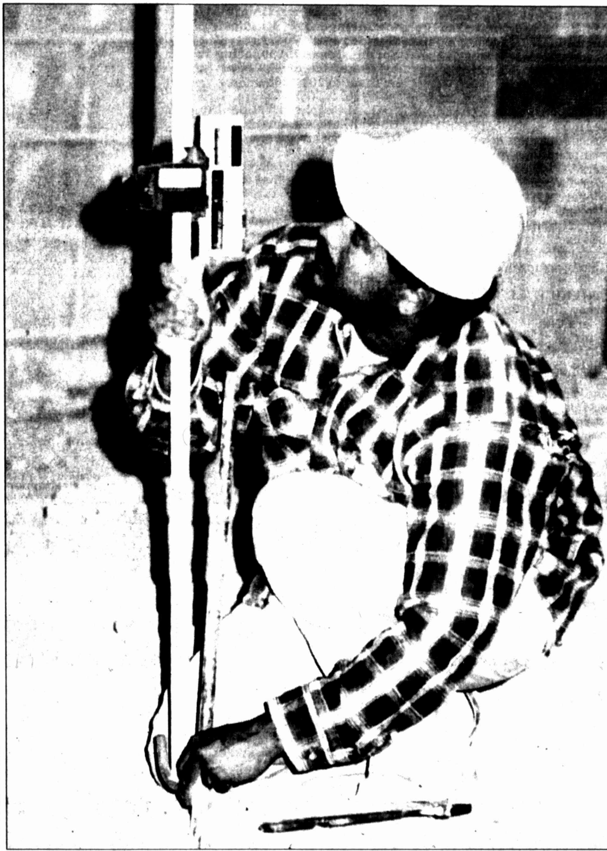
As construction on the new junior high continues Monday, Joe Solis, with Monterey Construction, grades the floor of a hallway to ensure that it is level.
