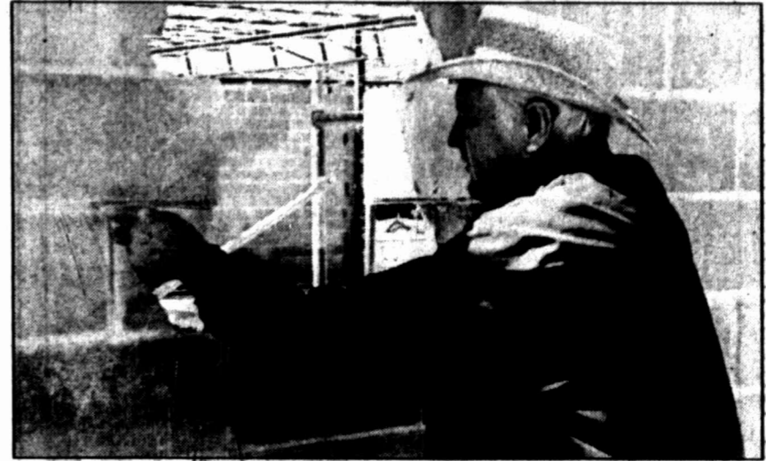
HERALD photo/Steve Reagan Ron Logback, BSISD assistant business manager, checks the condition of mortar at the city's new junior high school. The project is four weeks behind schedule because of problems with the mortar.
