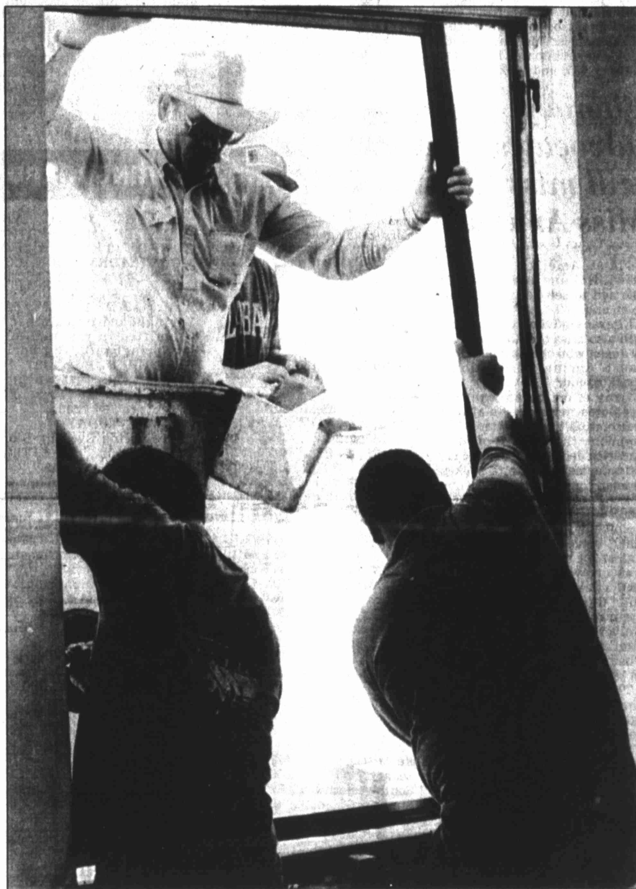
HERALD photo/Jonathan Garrett Ronnie Hipp (top left) holds the top of a window while standing in an outside basket with Tommy White while Domingo Rios (bottom left) and Rudy Gutierrez attach the window at the bottom. The four men were working over the weekend, installing windows in the Settles Hotel building.
