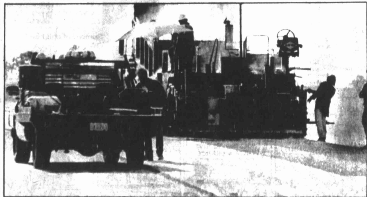
Howard County Road and Bridge Department crew members go about the business of sealcoating and paving county roads each summer, despite 100 degree temperatures. Crew members are seen here in northern Howard County and before the summer is over will have sealcoated and paved almost 60 miles of county roads.
