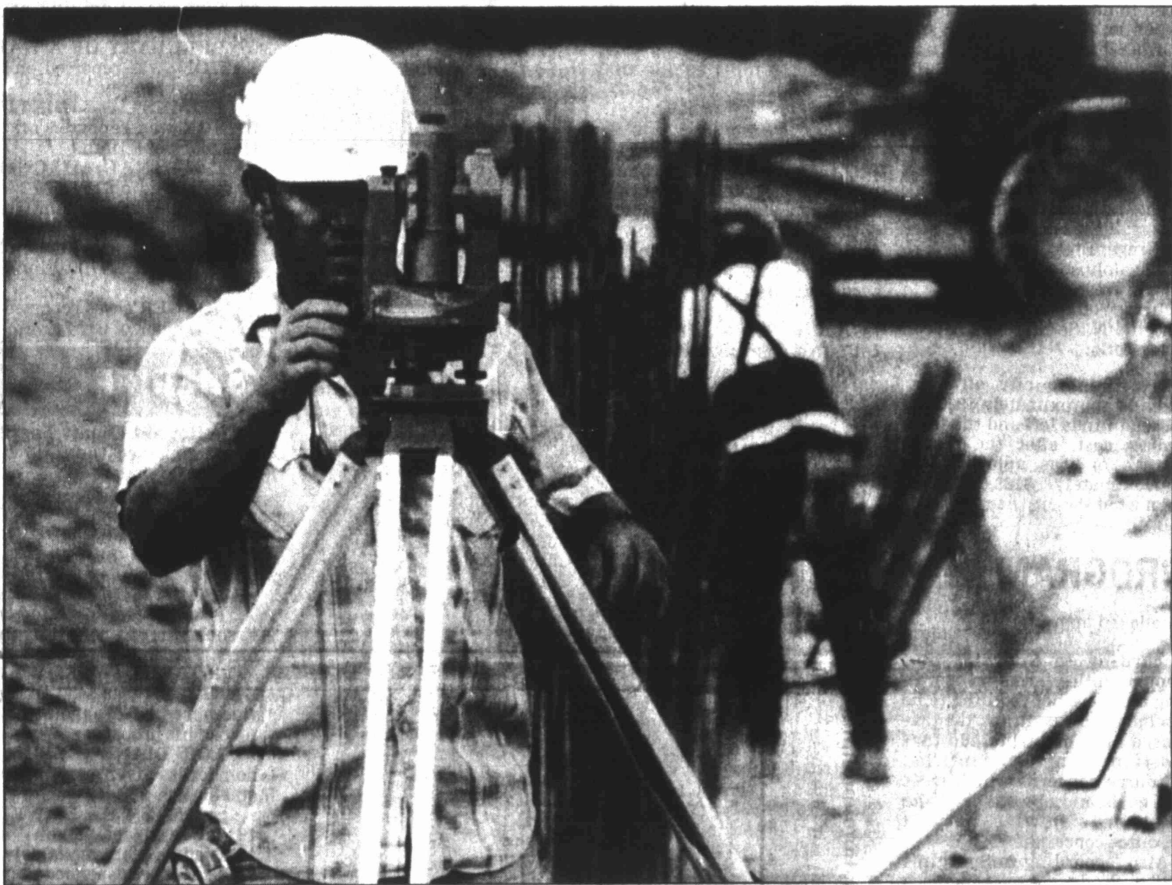
Ronny Smith uses a sextant to help workers line up foundation frames on the new junior high school being built on the site of the former Boydston Elementary School.
