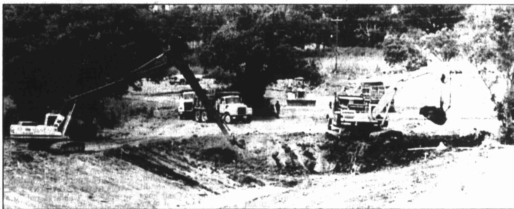
Dredging work on a new channel for Beals Creek, extending northwest from the Gregg Street Viaduct toward the old compress site, has been under way for the past week.
