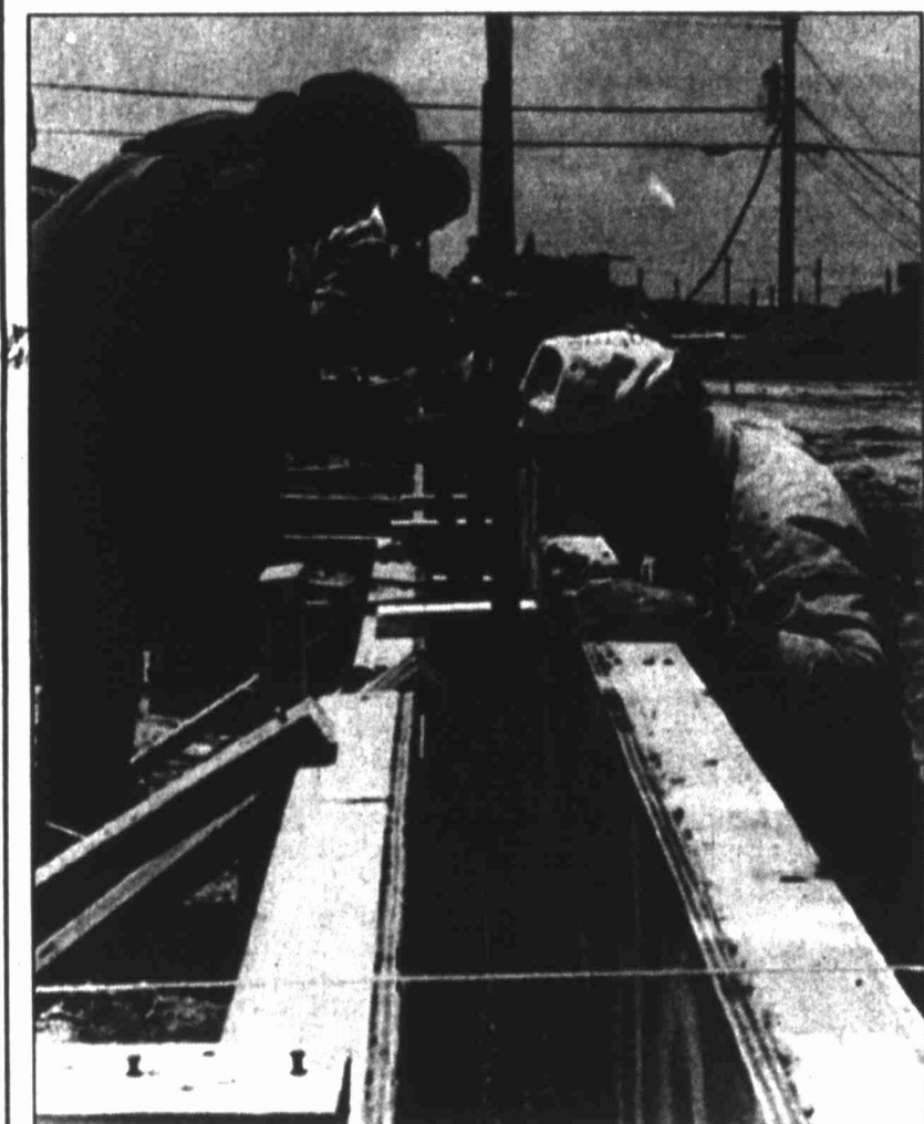
HERALD photo/Jonathan Garrett Work is continuing on the go-cart track at 11th and Scurry as Indio Munoz (left), Joe Silva, pouring concrete, and Hubert Barber, owner, work on the retaining wall to hold the dirt in on the track.
