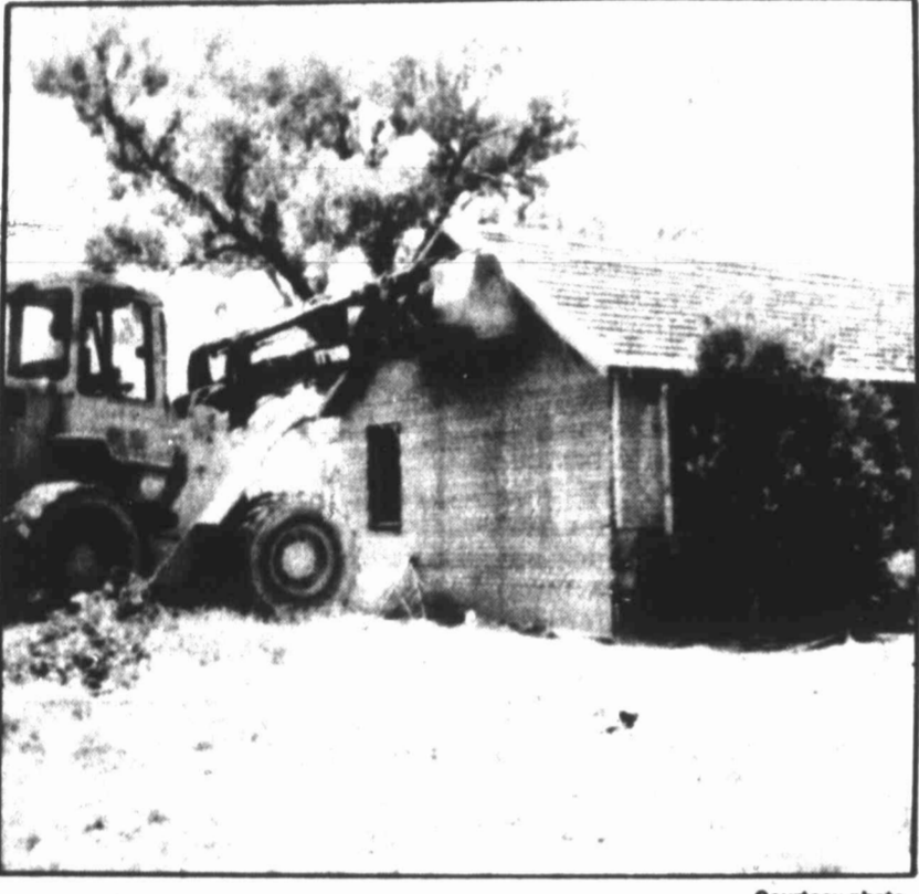
Courtesy photo The home of Odie May Sanchez at 1009 Sgt. Paredes St. is one of six homes to receive rehabilitation assistance as part of the city's HOME program. Mrs. Sanchez's home is being completely rebuilt as part of the program.
