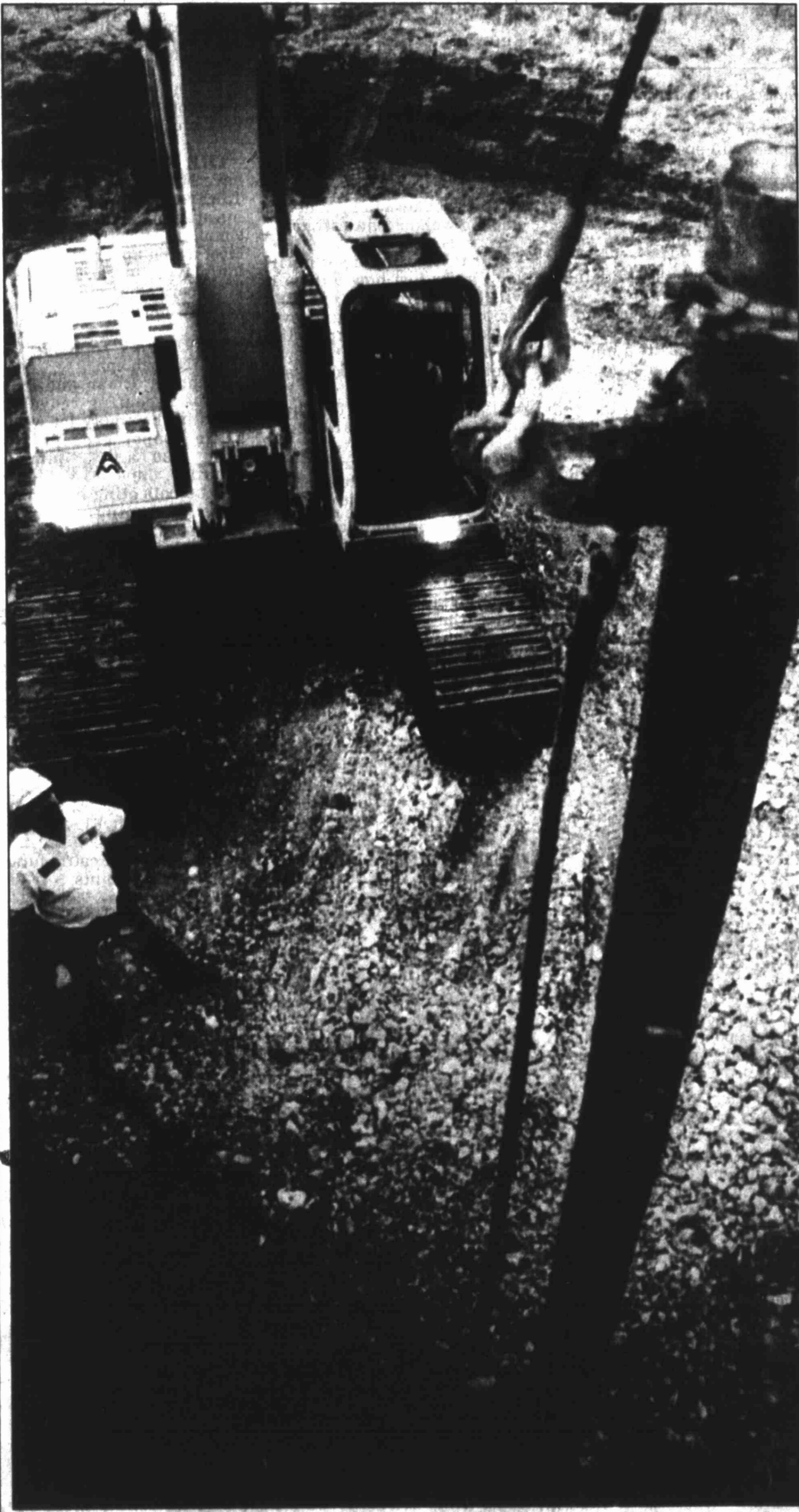
Rick Bolles directs crane operator Kenny Davis as city employees work to repair a broken sewer main located under the Benton Street Bridge. The 14-inch clay main collapsed as a water jet was being used in an attempt to unstop a clog.
