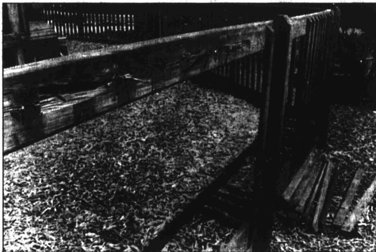
The wooden fence surrounding the Kids' Zone playground was among parts of the park vandalized last weekend. The Friends of the Park will have a work and repair session Saturday in an effort to repair the damage done by vandals, in addition to putting finishing touches to the park that include erecting a new swing.
