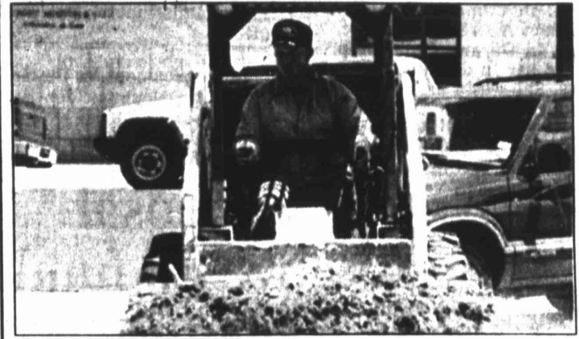
County employee Curtis White removes topsoil on the Courthouse lawn in preparation for re-sodding.
