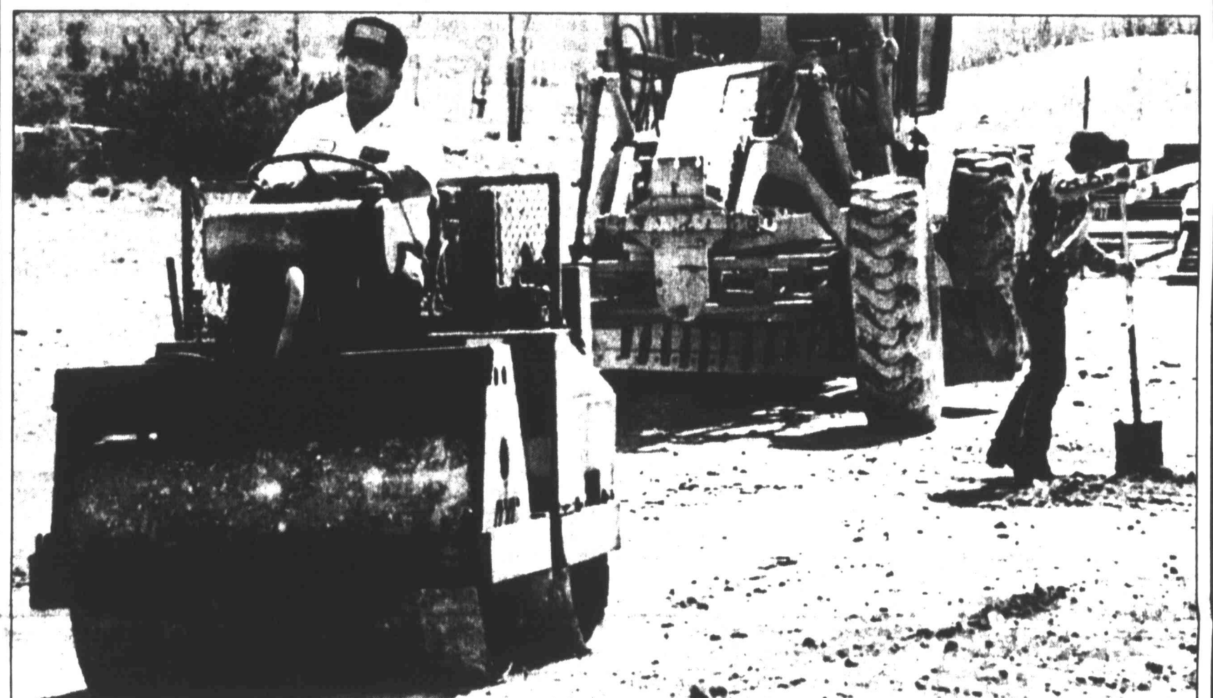
City of Big Spring employees Jesse Baker (left) and James Hoover work on the entrance at Comanche Trail Park, adding a new lane. The project was first envisioned by the Big Spring Area Chamber of Commerce. Construction is a cooperative effort between the city and the Texas Department of Transportation.
