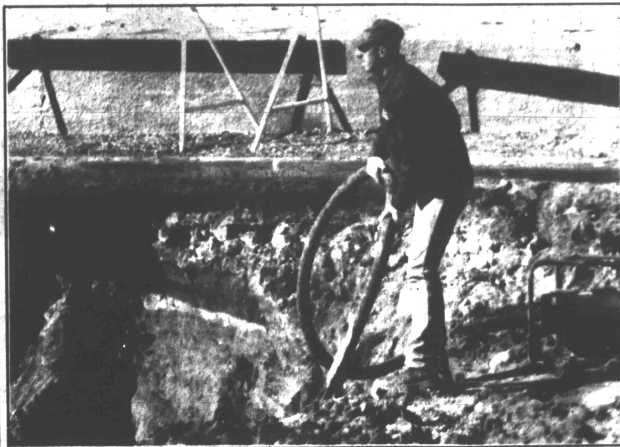
Chad Harber vacuums water out of a hole dug to replace old piping under the Union Pacific Railroad yard at 1st and Scurry. Officials plan to run smaller diameter piping through the existing line to avoid having to remove tracks in the rail yard.
