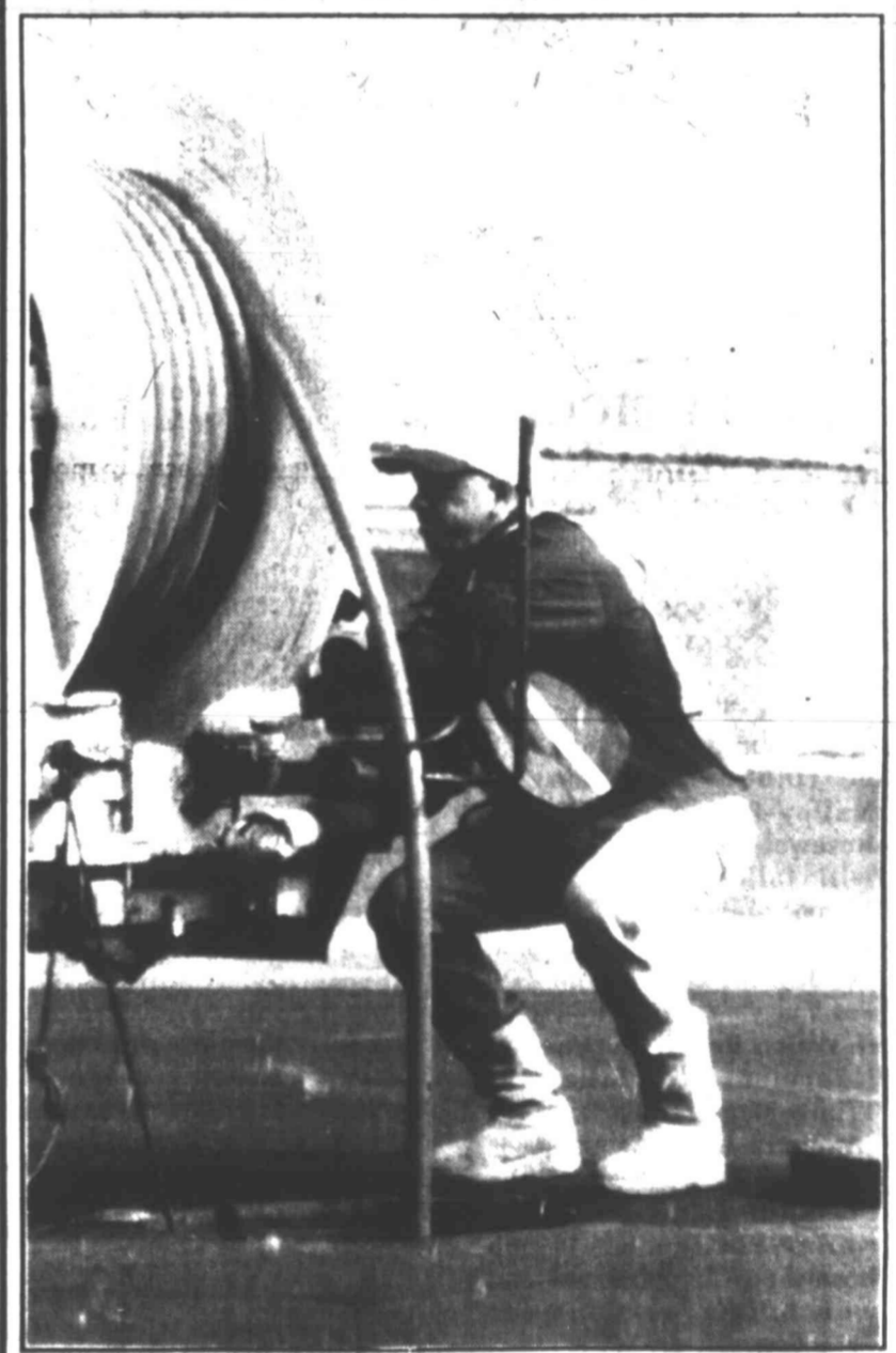
City of Big Spring employee Tony Bustamante encounters a rough time as he works on a sewer system problem on Birdwell Lane near Sixth St.
