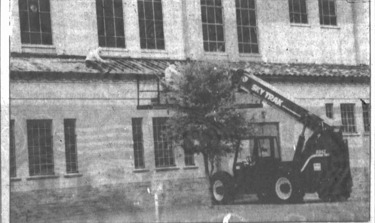
Because of the wear and tear it has taken through the years and because of hail damage received in May, the roof on the city's Municipal Auditorium is being replaced. The estimated cost of the two month project is $250,000.
