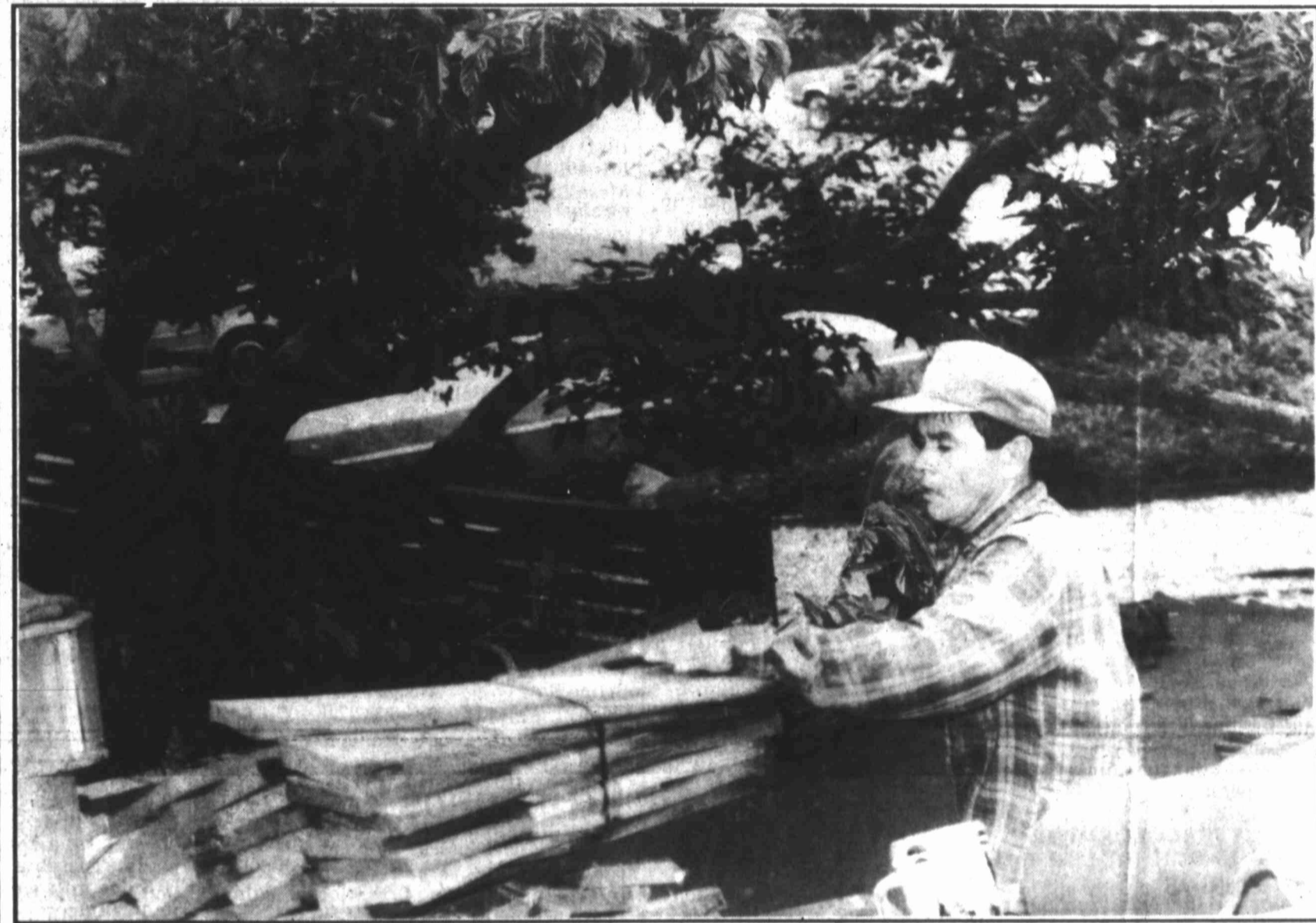
Fidel Menjilux carries shingles onto the roof of A.K. Guthrie's home at the corner of Osage and Indian Ridge. Menjilux works for Shaffer & Companies of Big Spring and says he's been plenty busy during the last couple of weeks.
