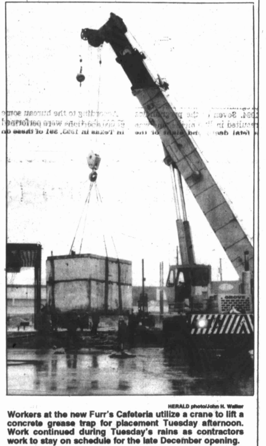
Workers at the new Furr's Cafeteria utilize a crane to lift a concrete grease trap for placement Tuesday afternoon. Work continued during Tuesday's rains as contractors work to stay on schedule for the late December opening.
