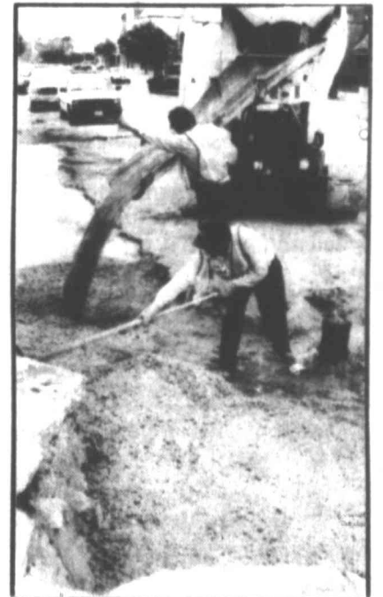
City of Big Spring workers spread concrete into a trench where they were working on a water line break this morning. The break and subsequent repair work has shut down Fourth Street next to the Howard County Courthouse, and is expected to remain closed until late Saturday.
