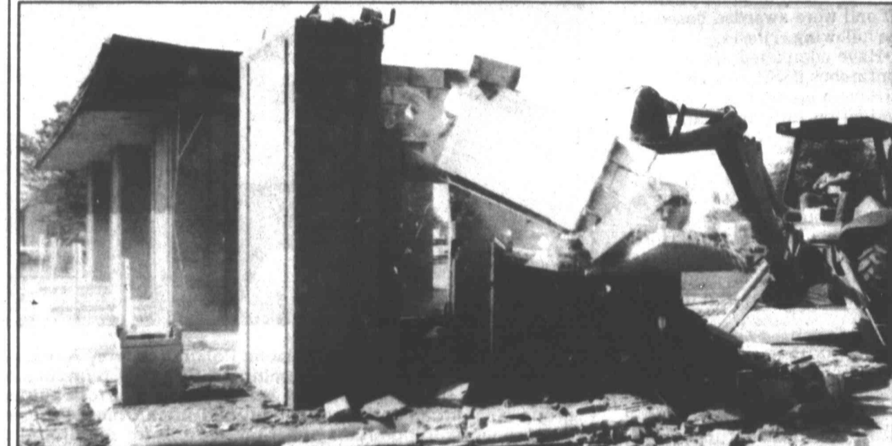
The recent construction at Security State Bank will be a thing of the past soon as new drive up windows are almost complete and should be operational sometime in September.
