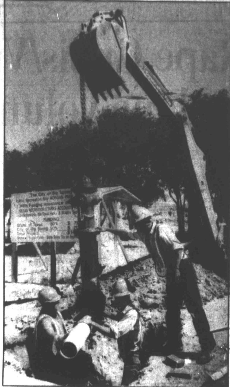
City of Big Spring workers drop a fire hydrant into place at the new Morgan Park recently. The city tapped into a nearby water line for both the hydrant and a newly-built park fountain.
