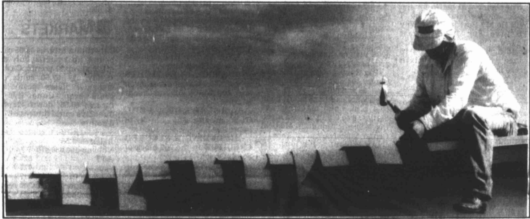
Tom Wilson of Five Star Roofing sits on the edge of a roof and hammers a shingle into place Tuesday. Many roofing projects are underway in Big Spring to repair damage done in May's hailstorm.
