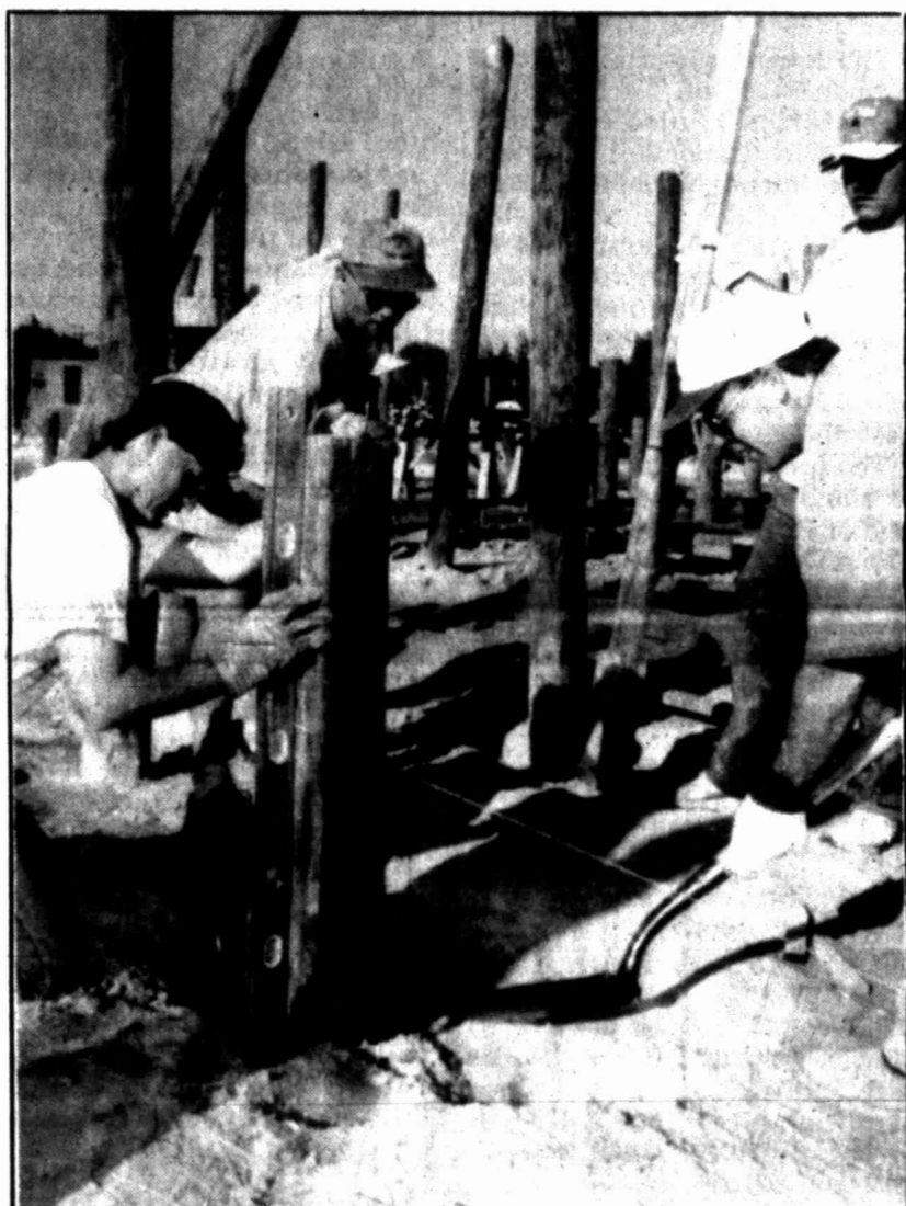
Volunteers measure, level and stabilize one of the dozens of posts that were being put into the ground Wednesday during the first construction day of the new Kids' Zone playground. The equipment is expected to be completed this weekend.
