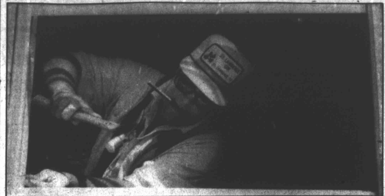
Steve Moses hammers a nail into sheetrock around a window frame during the annual Christmas in April project Saturday. Moses and other members of the Trinity Baptist Church were working on a house on East 11th Place.
