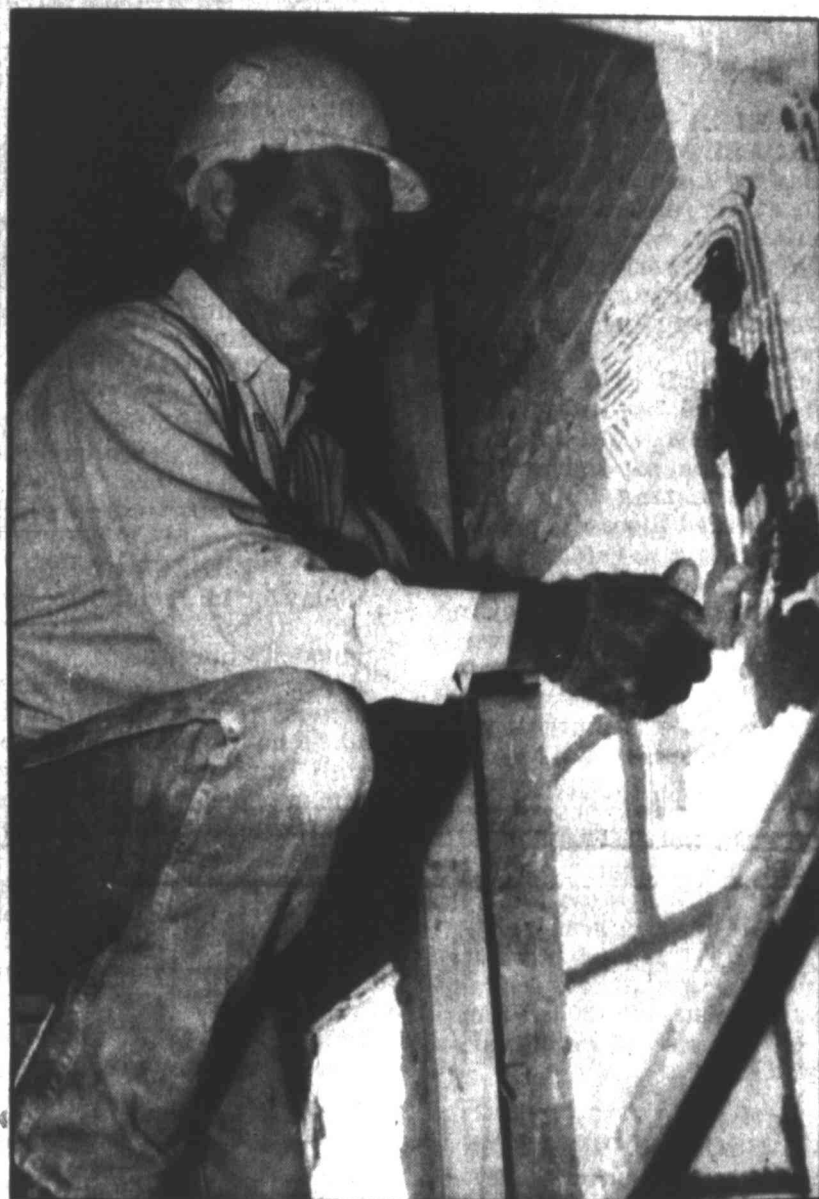
Jr. Nava places a cinder block into place as he and several other workers have been renovating the old Winn Dixie building Wednesday. Dollar General currently occupies one-third of the building, and the remaining area is being divided into half for future tenants.
