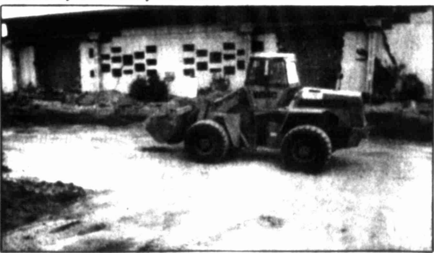
A front-end loader works behind the former site of Bluebonnet Savings and Loan, which will become the Howard County Library.
