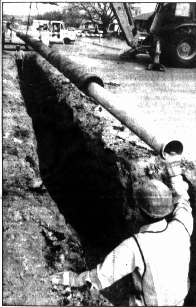
City of Big Spring crews put a water line into place across West 16th St. recently as part of a street renovation project. All water lines under the roadway are being replaced before the road construction begins in April.
