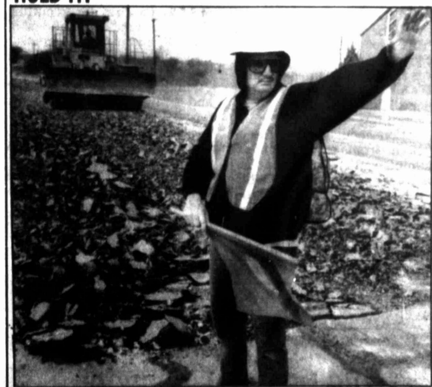
Steve Starr directs traffic while work continues on the Airbase Road rebuilding project in the background.
