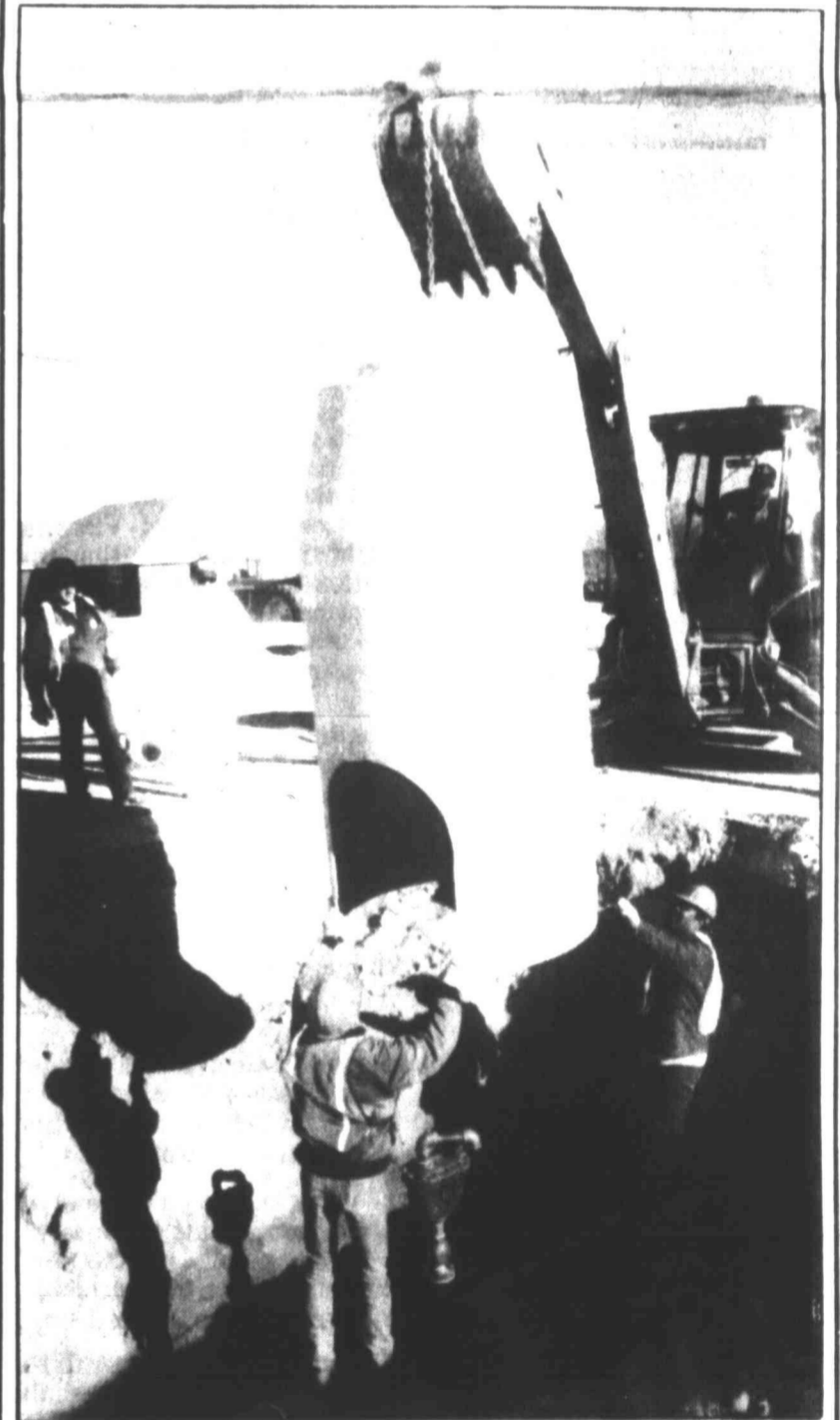
City of Big Spring workers lower a fiberglass manhole into a large pit on Baylor St. Wednesday. The covering was being fitted over a relief valve on a 20-inch main. Herald photo by Tim Appel
