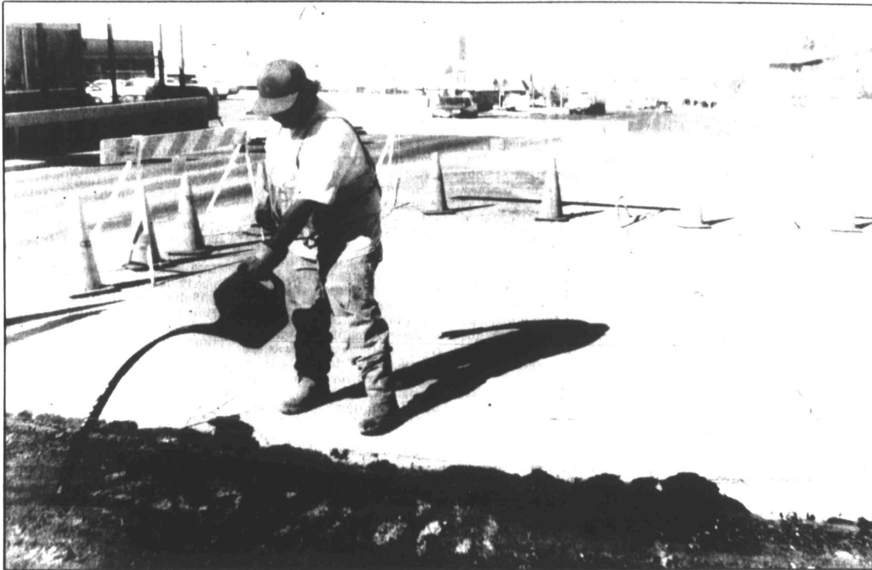
City of Big Spring worker Juan Pablo Mendez pours oil onto gravel before hot mix is applied on South Gregg Street Tuesday afternoon. The repair work, which closed the northbound lanes of Gregg Street, was due to a water break. Herald photo by Tim Appel
