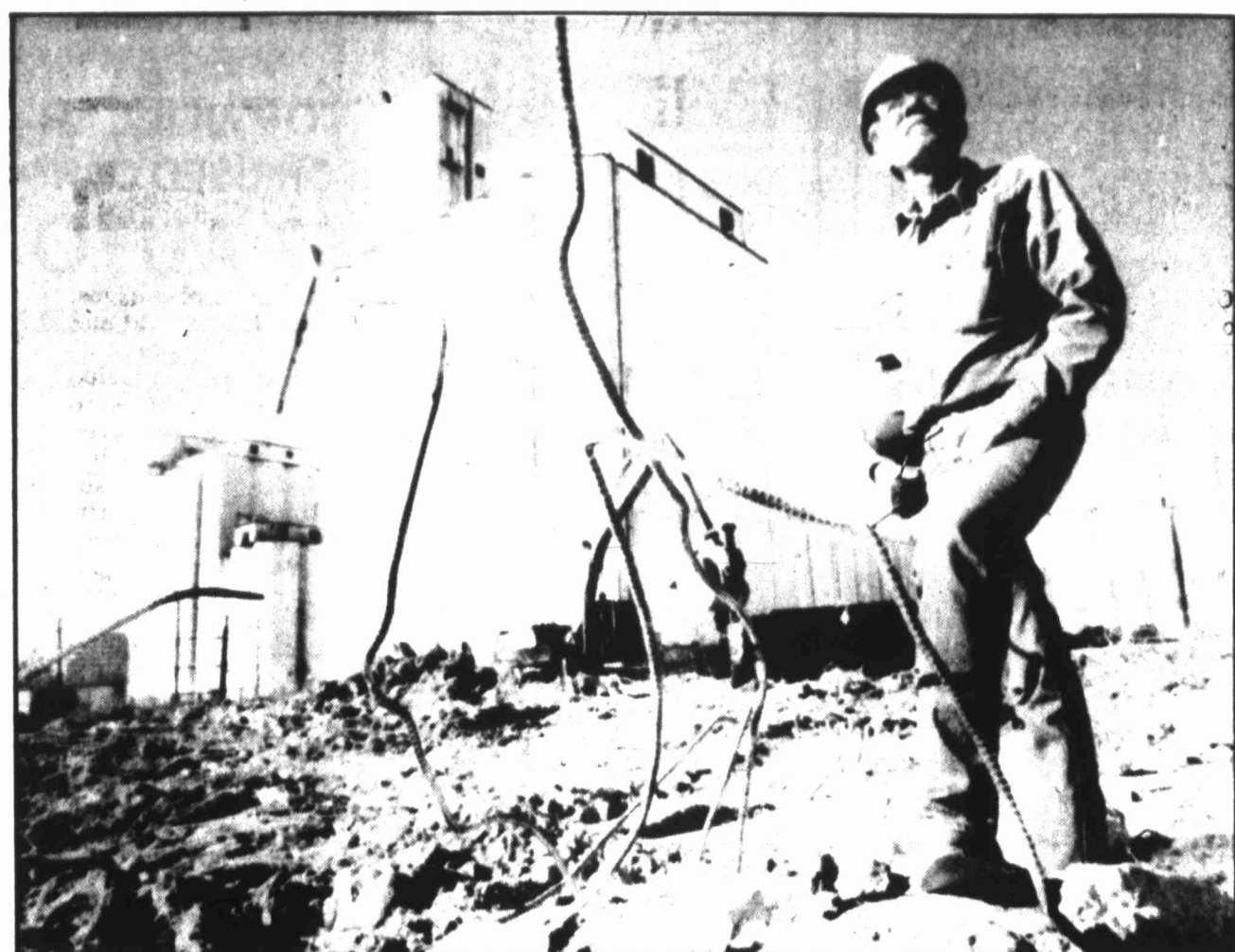
Demolition worker Bobby Kestner stands before the landmark rice silos on Memorial Drive in Houston. The 30-year-old edifices will be demolished over a period of time by wrecking ball and dynamite-fed implosions. Most of the debris will be recycled.
