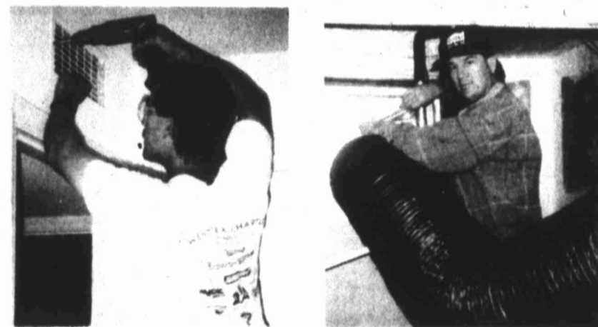
Mark Heinis and Rodney Ferrell prepare to clean a local air duct system.
