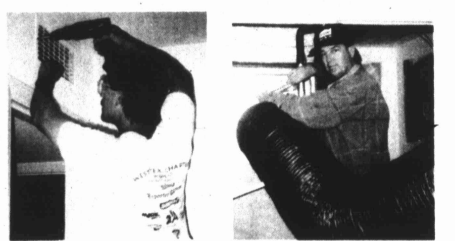
Mark Heinis and Rodney Ferrell prepare to clean a local air duct system.
