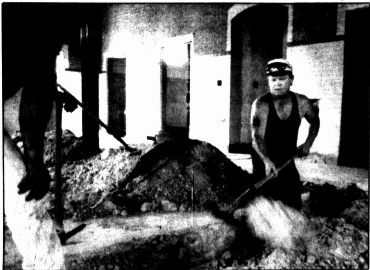
Randy Small digs a trench where plumbing will go on the first floor of the old downtown fire station Tuesday. Work has begun on the station, which will house the Big Spring City Council chambers in the near future.
