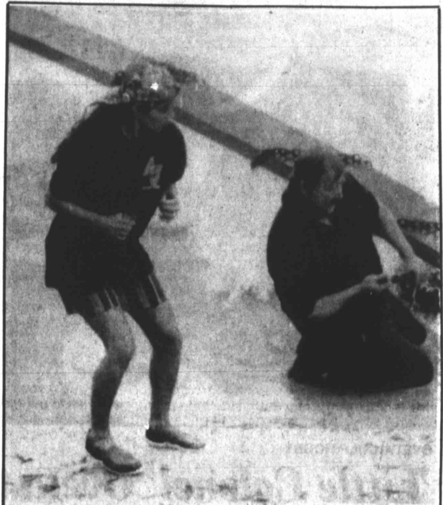
Danny and Kim Chaffin attempt to secure the cap of a new seawall as water slams up against it in Sandbridge, Va., Wednesday. Area residents were securing beach property as Hurricane Felix approached the coast. Felix, though, has decided to dawdle in the Atlantic Ocean and is expected to hit land Friday night.
