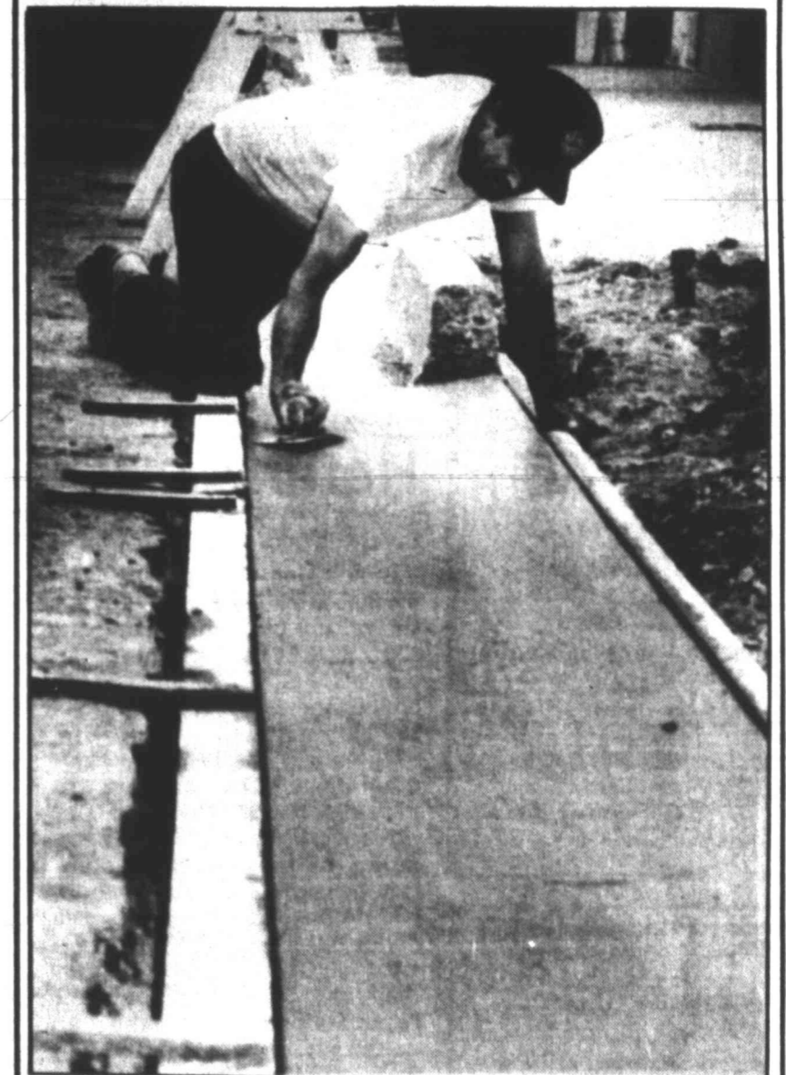
City of Big Spring worker Jorge Parra smooths out the concrete along Runnels St. between Third and Fourth streets recently. The concrete will be an expanded entrance to a driveway in the area.
