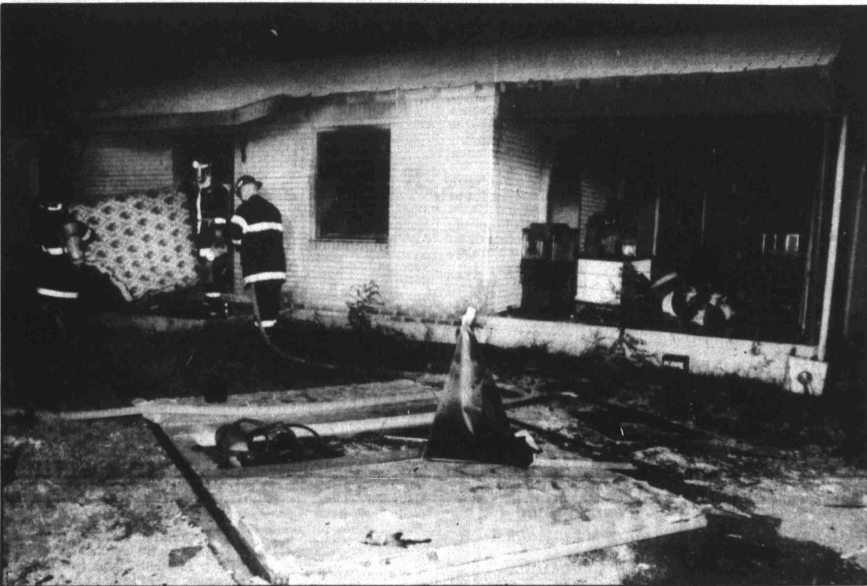
A wall from a converted garage at 3301 Abilene sits on the ground after being blown by an explosion Tuesday morning. John E. York was burned and taken to the hospital after being rescued by a neighbor and later transported to Lubbock.
